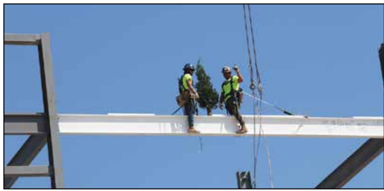
Construction workers place the final beam on top of the new Muscogee (Creek) Nation Citizen Services Building. April 14, 2025. Okmulgee, Okla. (Braden Harper/MM)
